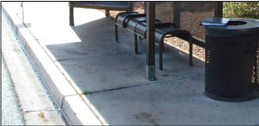
Bus stop obstructing the sidewalk
