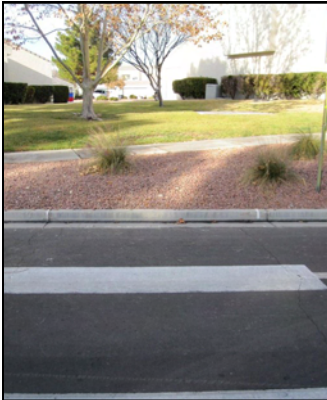
Crosswalk at Lake North and Waterview Drives without a curb cut to the sidewalk
