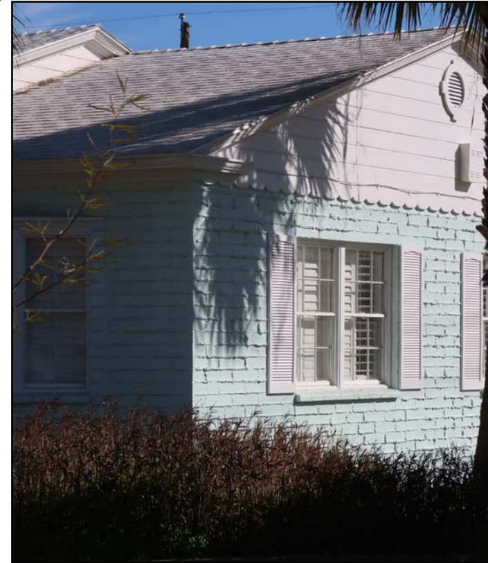
Image 19: Example of weeping mortar.
