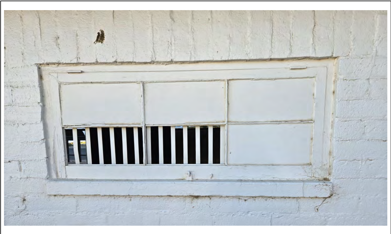
Office/Stables – North elevation window detail Kautz Environmental Consultants, Inc., November 2024
