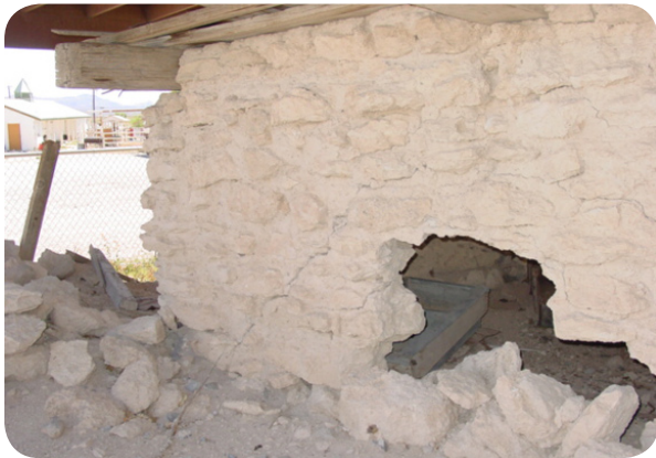
Caliche Stone Hut. John Herbert Nay, the first known owner of Tule Springs in recent history, constructed this caliche stone hut which is in dire need of preservation work.
