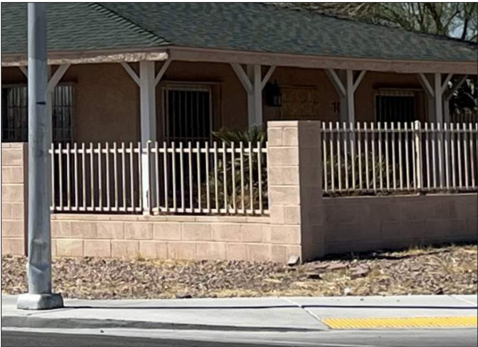
Wrought iron fence with CMU stem wall
