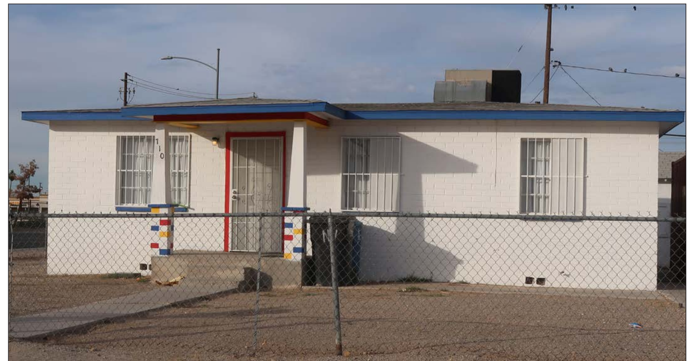
Recommend placing MEP at rear slope and not street-facing elevation
